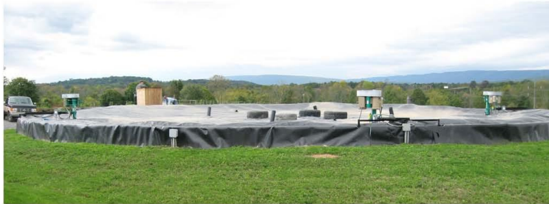
Complete Mix digester with non-expandable flexible cover.
