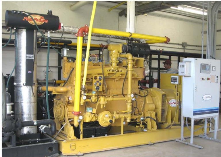
G342 Caterpillar, 1200 rpm engine with 250 Volt, 1 phase generator.
