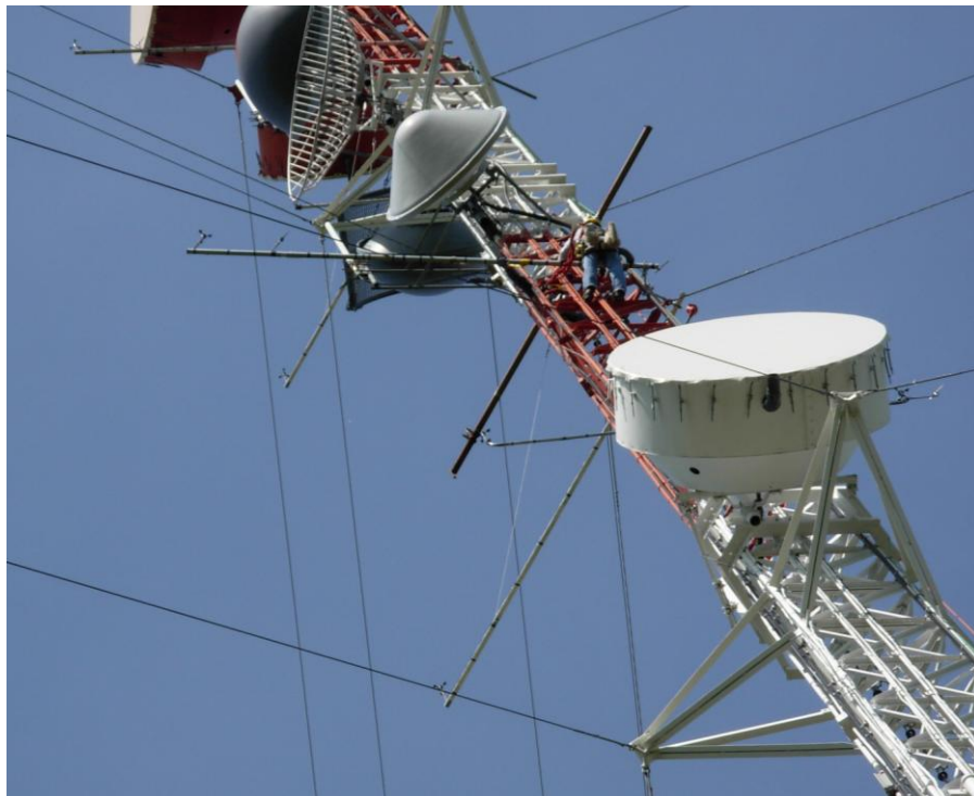
Figure 17: View of FirstEnergy Tower and Microwave Dishes during installation activities at Lorain
