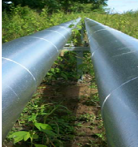
Figure 3.2: Typical above ground insulated pipe installation
