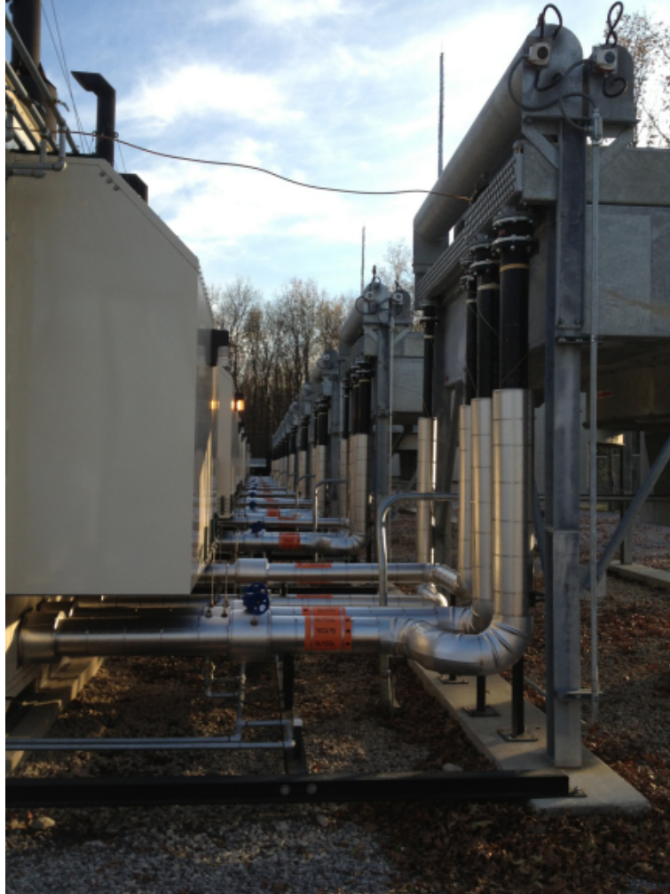
Figure 2.1. Engine-Radiator Piping System at EDI
