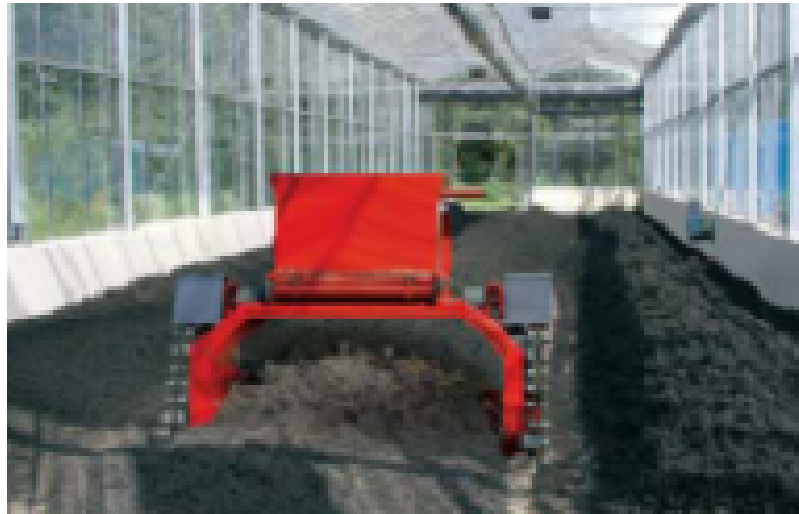
Figure 4.7. Solar biosolids drying greenhouse with agitation unit
