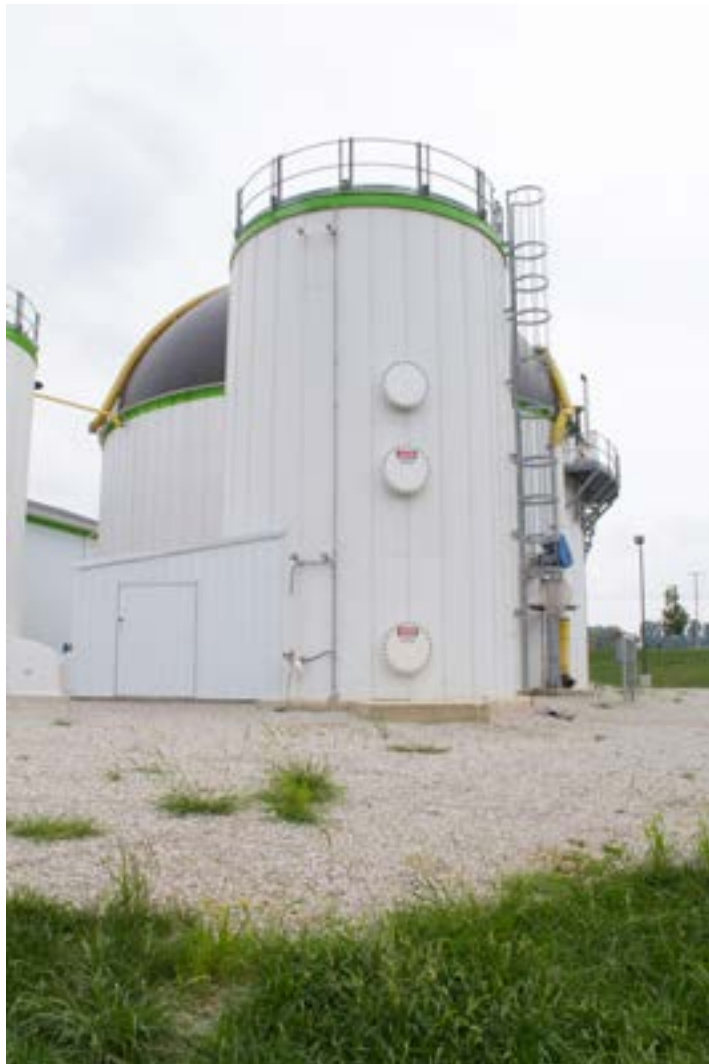
Quasar Energy Partners anaerobic digester at the Ohio Agriculture Research and Development Center.
