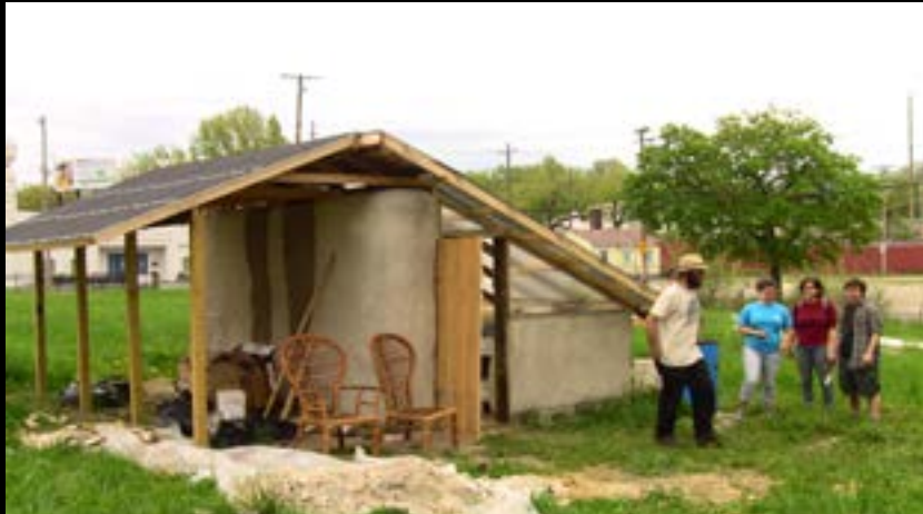
A strawbale greenhouse provides a space for seedling starts and vegetable production at Vel's Purple Oasis in Cleveland. The straw-bales provide insulation to improve heat retention during cold months. The greenhouse was built over a weekend by 80 volunteers, including students from the nearby John Hayes high school.
